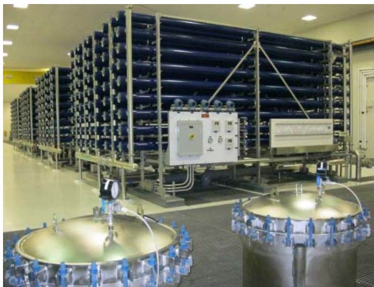
North RO Plant Production Trains
